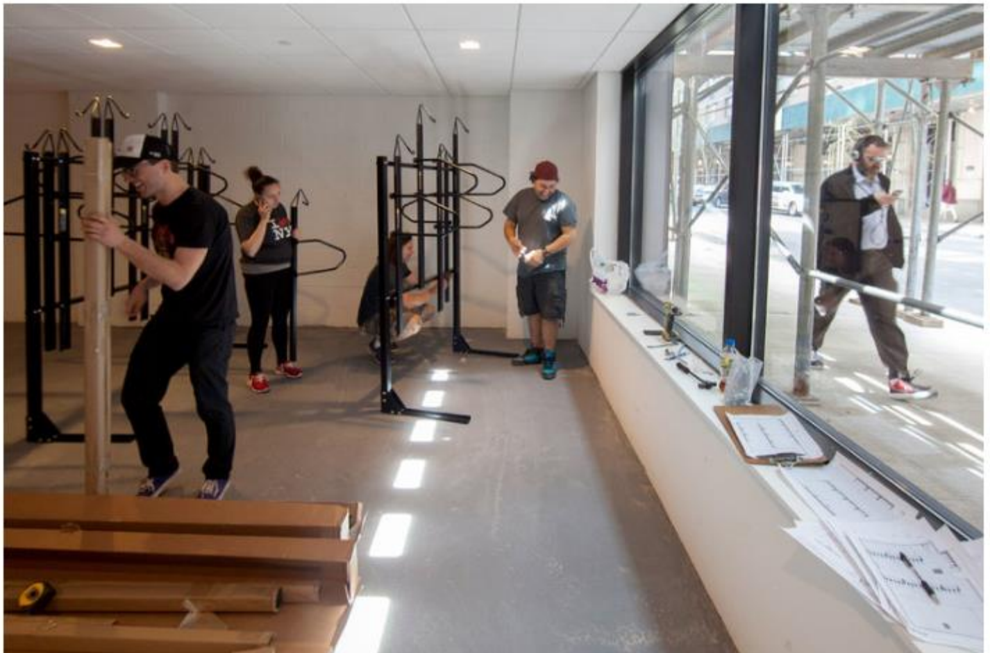
Bike storage racks are installed at 535W43, a luxury rental building nearing completion on West 43rd Street. Dave Sanders for The New York Times
